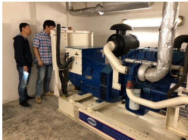
Figure 8 The uninterruptible power system (UPS) and backup generators were examined during the exercise of power system failure.
